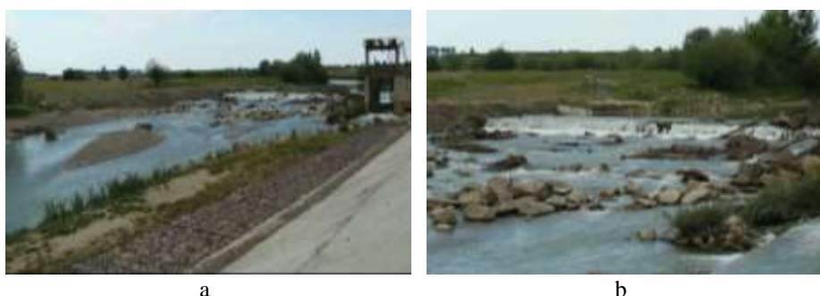
Fig. 5 – The current state of the catchment area: a - general view; b - detail regarding the energy dissipation basin at the bottom threshold.
