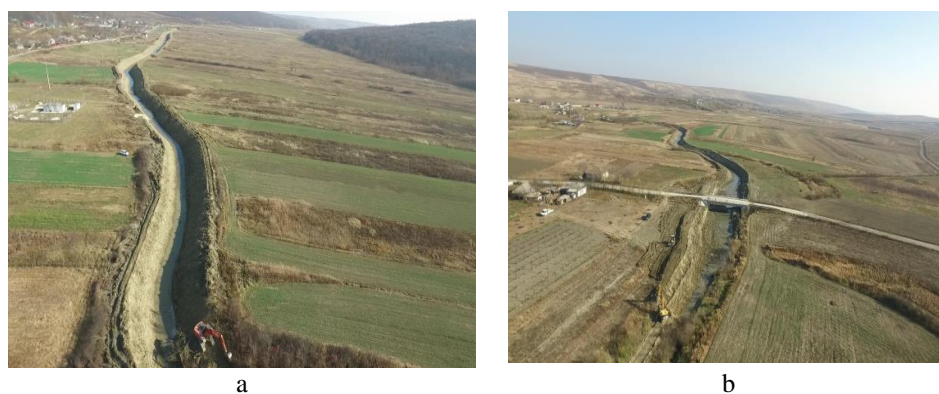
Fig. 4 – Overview of the transport capacity insurance works on Miletin River, Coșula commune, Botoșani county, year 2018 (A.B.A. Prut–Bârlad, 2018).
