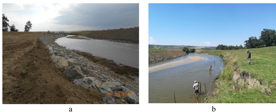
Fig. 3 – General view of the redevelopment works Bârlad River, Ghidigeni comm., Galați county, year 2018: a - consolidation of the left bank overgrowth; b - consolidation of the right bank loan prism (A.B.A. Prut–Bârlad, 2018).
