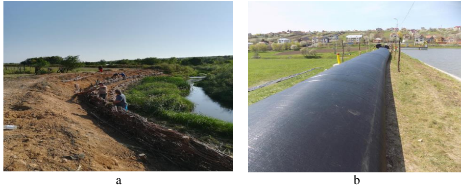
Fig. 5 – Overview of protection works on the Suhu River, Slobozia Conachi, Iași County, year 2018: a - vegetative consolidation; b - overhanging dams with the help of hydrobarages (A.B.A. Prut–Bârlad, 2018).
